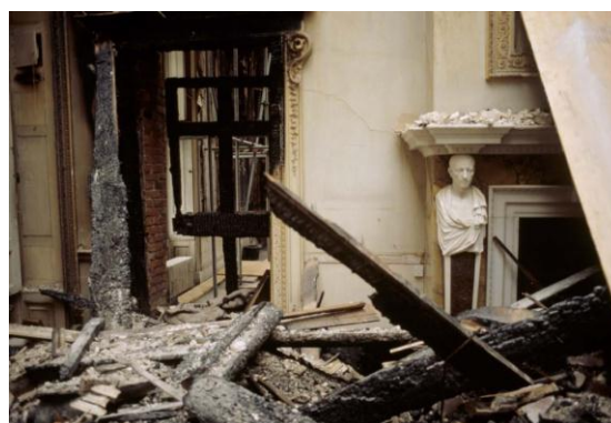
Fire damage in The Saloon following the fire at Uppark, the National Trust's 17 th property in West Sussex
